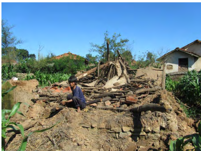
Totally collapsed house in Sinyang-ri, Yonan county, south Hwanghae province. The accumulated effect of years of poor maintenance, aggravated by strong winds during a typhoon at the end of June, as well as extended heavy rainfall have taken its toll on over 3,000 houses so far. Photo: Kamal Niraula/IFRC
