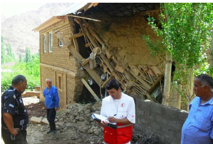
Rapid assessment of the damaged houses in Asht district. Photo by: RCS Red Crescent Society of Tajikistan
