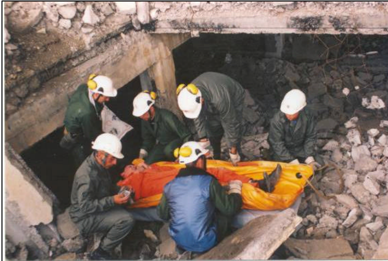
A reliable partner: Red Cross rapid response team helps people trapped in a building that collapsed in Gyumri.
