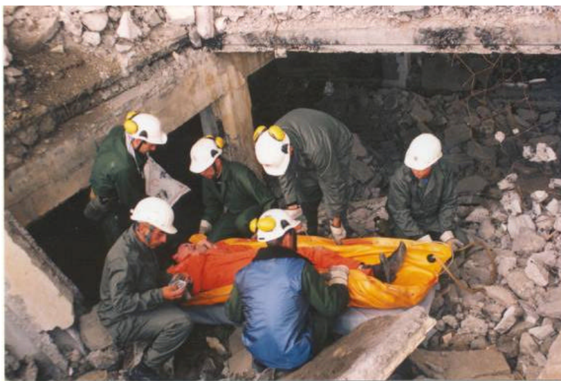
On hand: a Red Cross rapid response team helps rescue people trapped in a collapsed building in Gyumri.
