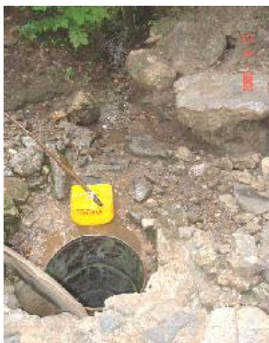
A traditional well in Mbuji-Mayi, eastern Kasai province (before rehabilitation work started).
