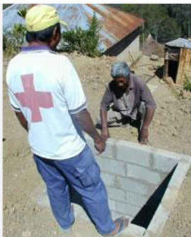
Crispin Baptista builds a latrine with technical advice from Red Cross plumber Afonso Alves
