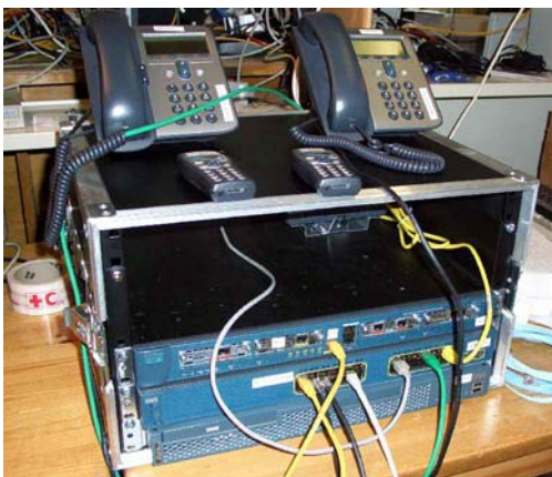
Prototype components mounted in frame. Note wireless and fixed IP phones.
