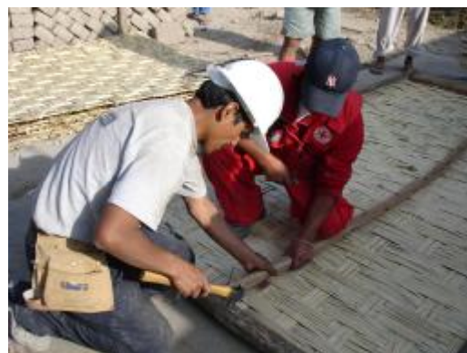
The Peruvian Red Cross Society volunteers and local communities constructed transitional shelters together using traditional materials, following the Pisco earthquake in August 2007. International Federation
