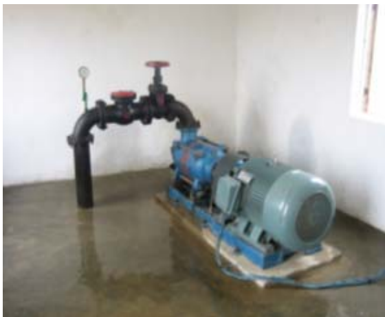
A pump installation in Sangbuk-dong, Mundok county.
