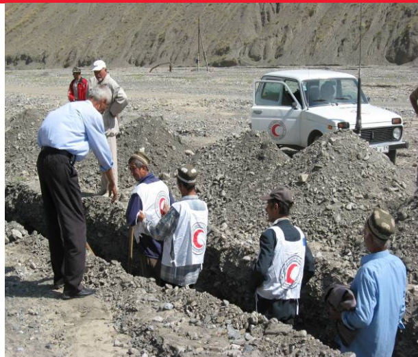
Water committees mobilized their community members to trench the main water piping.
