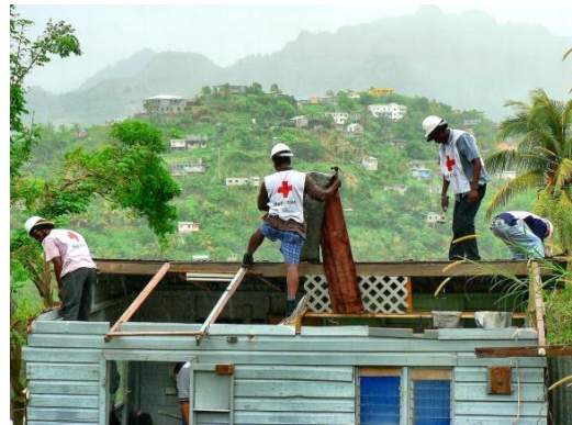
In November 2010, the Saint Vincent and the Grenadines Red Cross (SVGRC) volunteers repaired and replaced roofs lost after Hurricane Tomas struck the islands. Source: SVGRC
