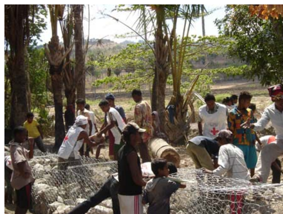
Community volunteers build stone barriers to protect from coastal erosion in Timor-Leste. (Photo: CVTL/IFRC)
