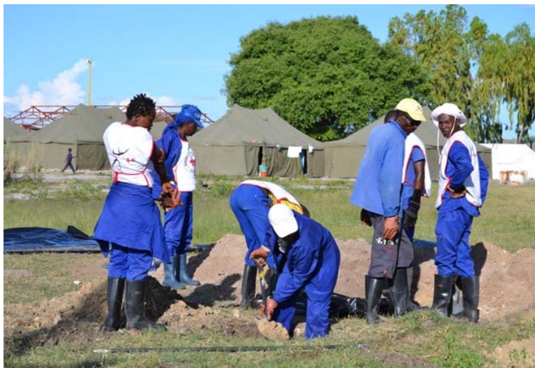
Namibia Red Cross volunteers preparing to erect a pit latrine at the relocation camp in Caprivi region, for utilization by families displaced by floods (photo: NRCS)
