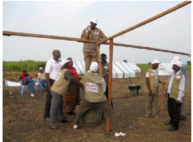
Red Cross of DRC volunteers conduct shelter construction exercise during the NDRT field training in December 2009 and January 2010 Photo: Red Cross of DRC
