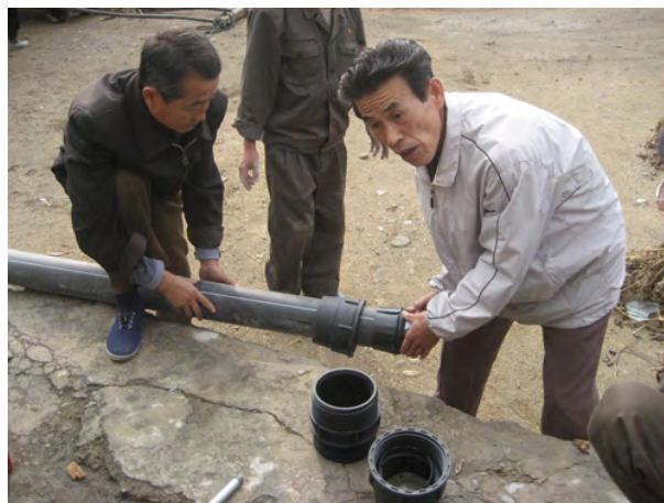
DPRK Red Cross water and sanitation technician is checking the quality of the delivered materials for the pipe laying of the water supply scheme Kim Ikson/IFRC DPRK
