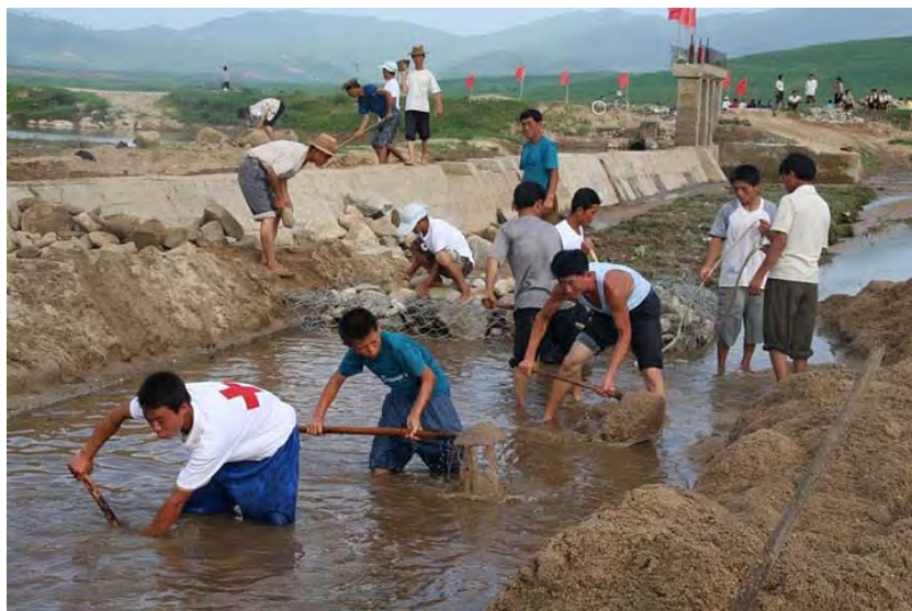
Community volunteers help with the construction work of a flood-mitigating reinforced riverbank in South Hamhung province. Francis Markus/IFRC
