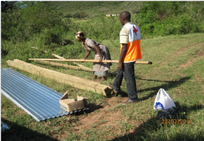
Red Cross volunteer assists a survivor of a hailstorm off load and store relief items for reconstruction
