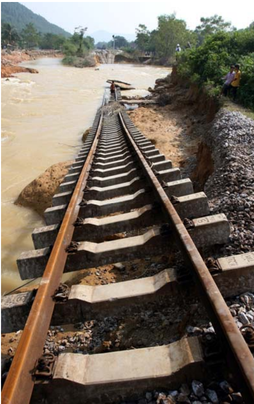
National railways badly damaged by consecutive flooding in Ha Tinh province Photo: Quang Tuan/ VNRC
