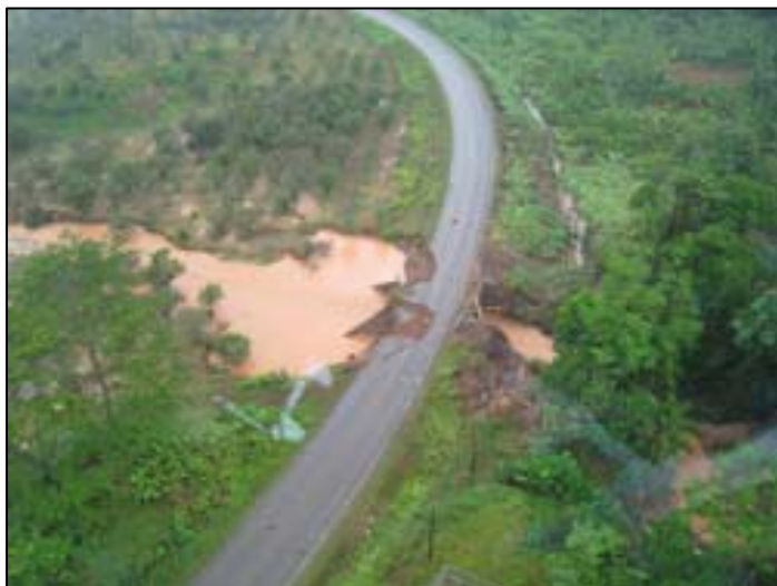
Damaged roads in Belize. Source: Ministry of Foreign Affairs, Belize.
