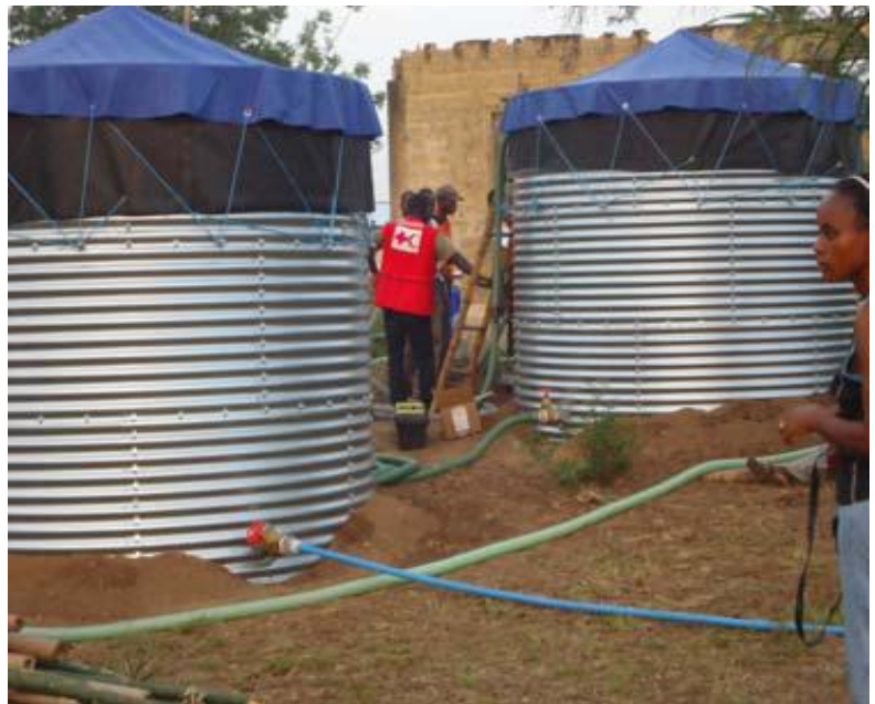
Water supply facility (Kit 5) installed by LNRCs trained volunteers and staff at Bortuo in Liberia. Photo IFRC
