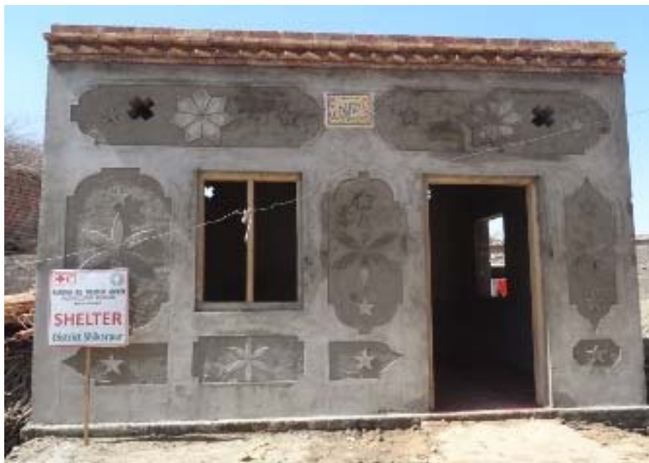
One of the houses built under the shelter cash grant programme in Shikarpur district, Sindh province. Photo: IFRC
