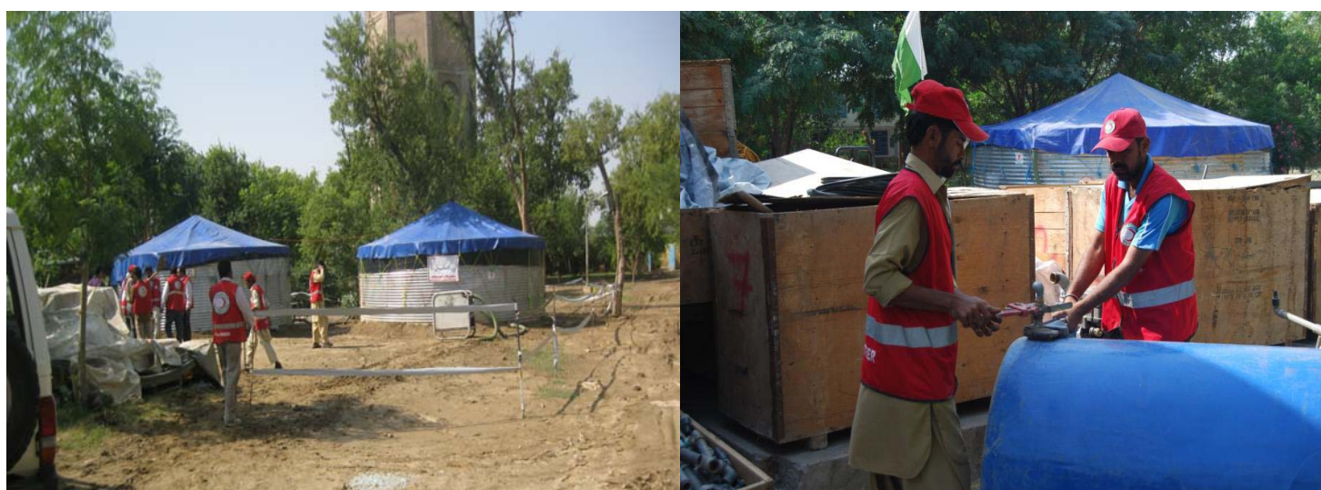
Water units installations in Jacobabad, Sindh Province (left) and D.G Khan, Punjab Province (right). Photo: IFRC
