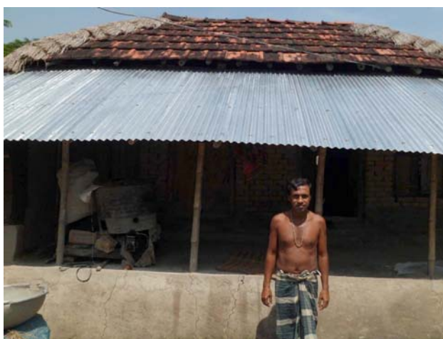
Shopon Kumar Mondol of Mesherdanga village of Satkhira district received cash grant to restore his damaged house. He brought some shelter materials and fixed the damages to prevent from heavy rain and provide a safe and secure place to live for him and his family. Photo: BDRCS volunteer.
