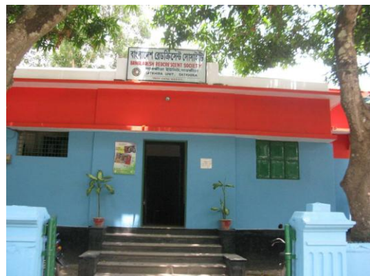
Renovation of BDRCS Satkhira unit office, part of which contribution is made from the emergency appeal. Photo: IFRC
