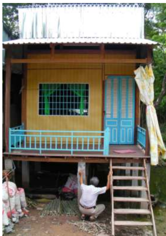
A regular visit paid by VNRC staff to construction site to ensure quality and progress of the work within project timeframe.
