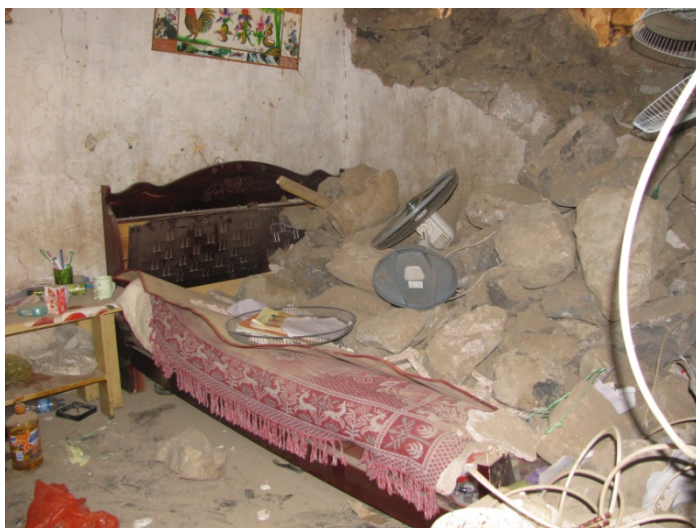
A house badly damaged by rolling rocks caused by the earthquake.
