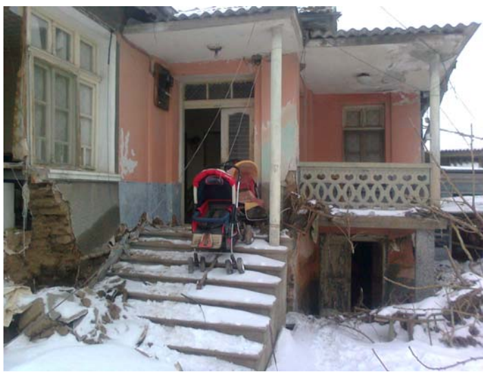
Family home damaged by extreme winter conditions Photo: Bulgarian Red Cross
