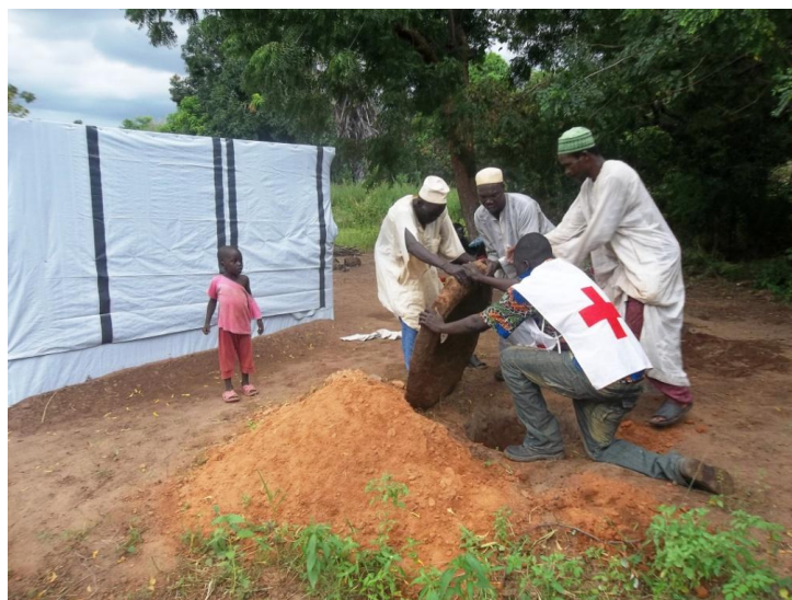
Cameroon Red Cross volunteers constructing emergency latrines in Northern Cameroon with assistance from members of the floods affected community / Photo by Cameroon Red Cross
