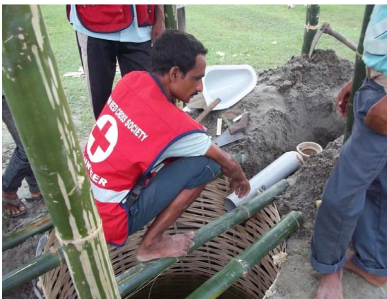
Indian Red Cross Society staff and volunteers constructing a toilet in Assam. Photo: Indian Red Cross Society.
