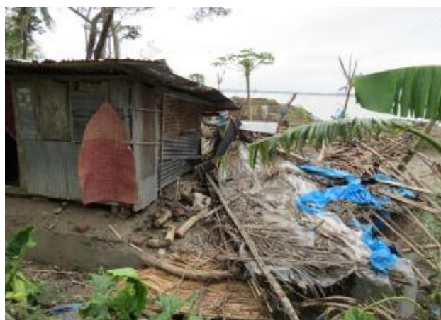
Shelter damage due to cyclone Mahasen. Photo: BDRCS.
