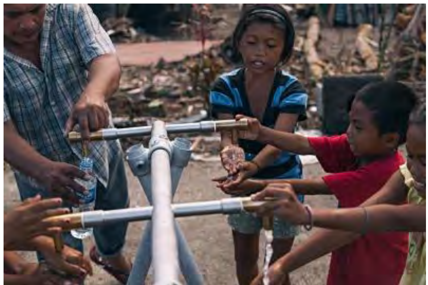
Water point installed in Tolosa (Leyte) by water and sanitation team
