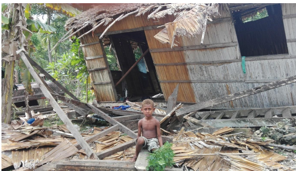
A child sits in front of his destroyed home in Radefasu village in Malaita, one of the communities in the Province that is also affected by the magnitude 7.8 earthquake that struck the Solomon Islands on the early morning of 9th December 2016. (Photo: SIRCS)
