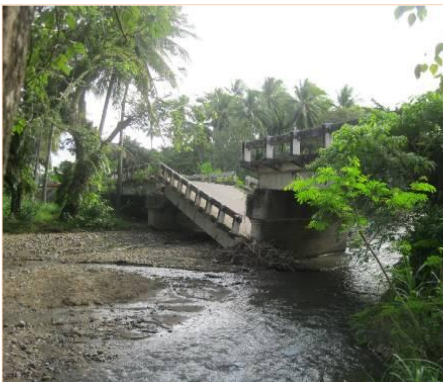
Jimalalud, Pangaloan Bridge: The quake damaged houses, bridges and critical infrastructure such as electricity and communication lines.
