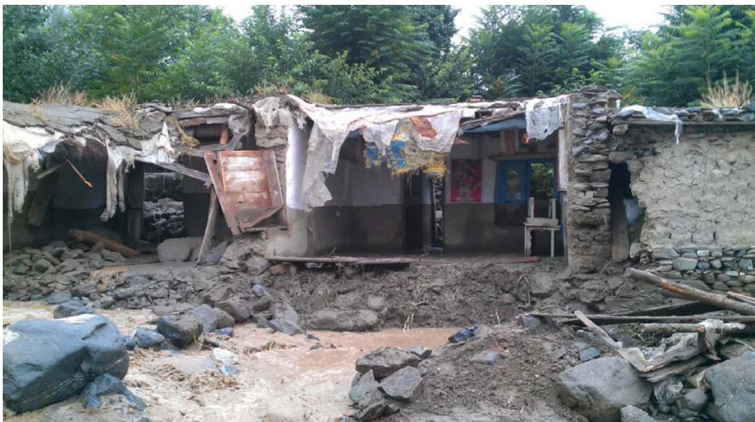
A house in Drosh area of Chitral district, KP province, partially destroyed by the flood. Photo: PRCS.
