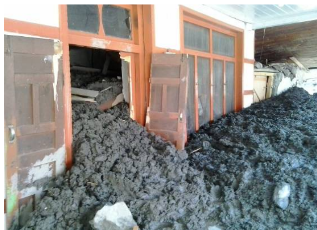
A house in Chitral district of KP province destroyed by silt from the overflowing river. Photo: PRCS.
