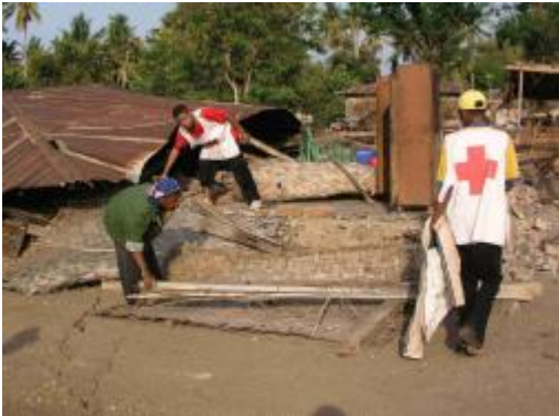
PMI local SATGANA volunteers help a single mother to identify some useful housing materials for further utilisation.
