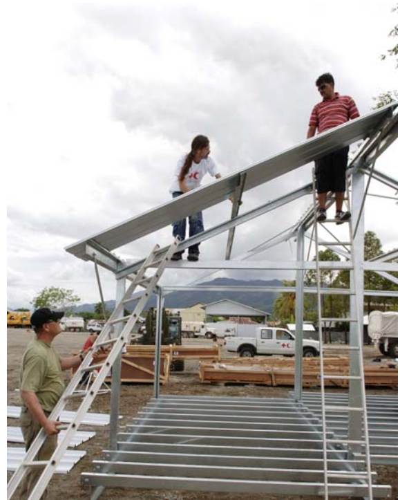
Galvanized steel frames being erected on first batch of the 20,000 transitional shelter units being provided in Indonesia.
