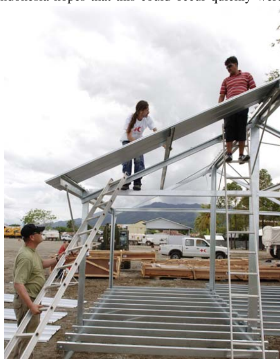
Galvanized steel frames being erected on first batch of the 20,000 transitional shelter units being provided in Indonesia.
