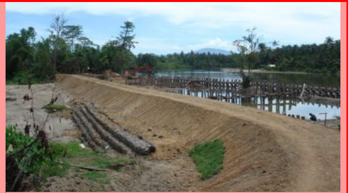
The Danish Red Cross dike is 210 metres in length using 1,956 cubic metres soil, 324 metres of wooden crib structures, 369 cubic metres of gabion structures and 1,400 square metres of Vetiver grass plants. This photo shows the dike near completion, when grass planting had just started. Danish Red Cross/Hans Hausmann.
