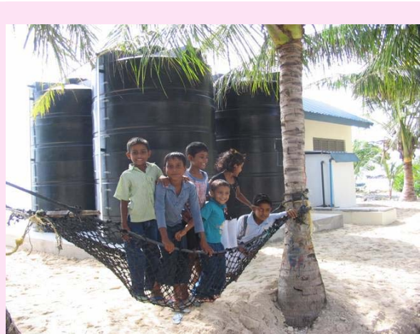
Happy children play in front of the newly installed supplementary water supply system on Gadhdhoo
