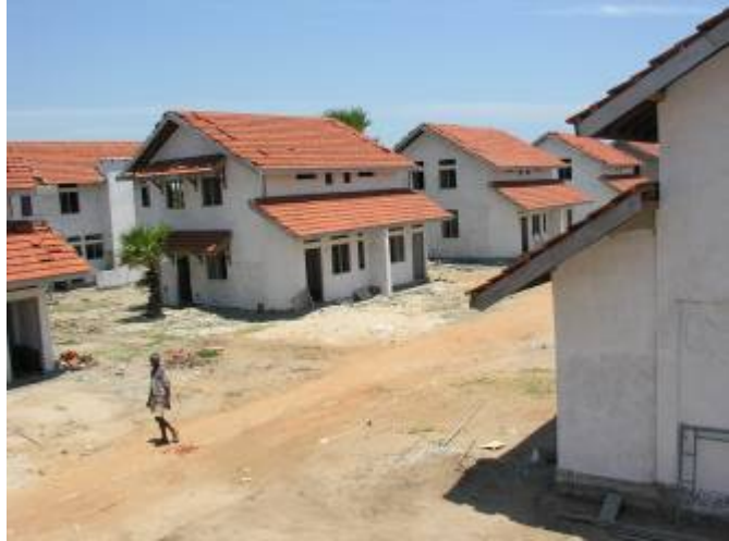
Houses nearing completion in the Ontachimadam site, eastern Sri Lanka. Beneficiaries are expected to occupy these houses by the end of December 2008. International Federation.
