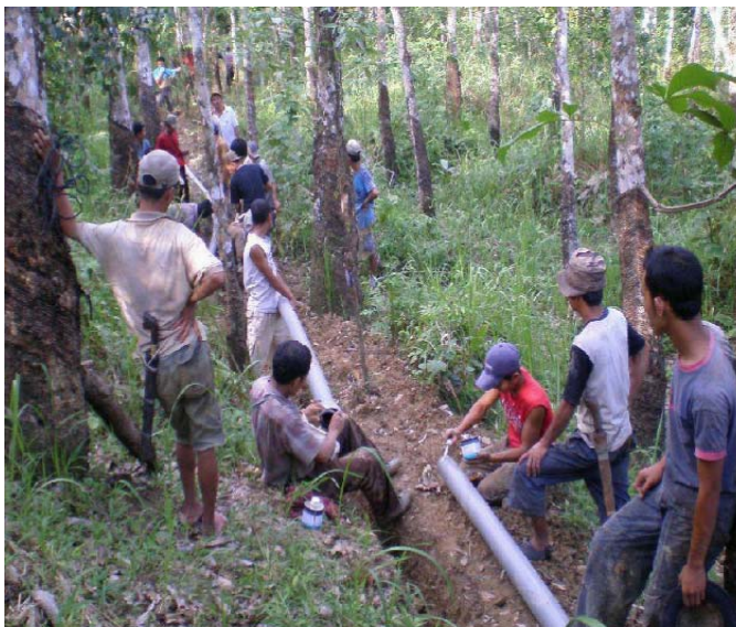
Gotong royong which means community cooperation is widely practised in Indonesia. In Nias Island, communities dig trenches in villages as part of the water and sanitation programme. International Federation.
