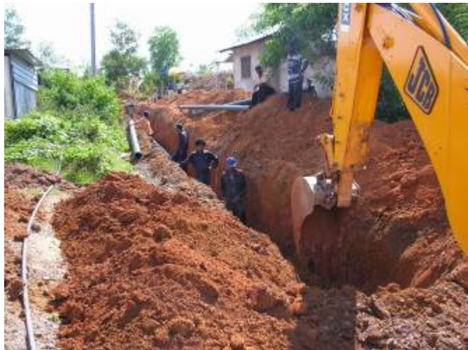
Trenches like this are being dug to lay pipes to provide safe water to new housing settlements in Ampara, eastern Sri Lanka. International Federation.
