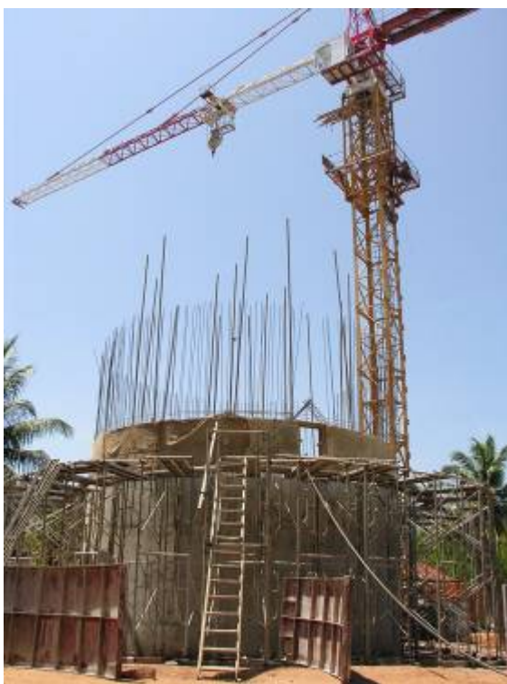
The construction of the water storage tank in Pottuvil, Ampara district which is implemented and supported by the IFRC and SLRCS and funded by the Irish Red Cross.
