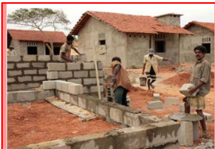
Construction labourers lay cement blocks to construct the wall of a CRRP house. Red Cross Red Crescent partners have channelled USD 50 million into owner-driven housing through the CRRP programme. International Federation.
