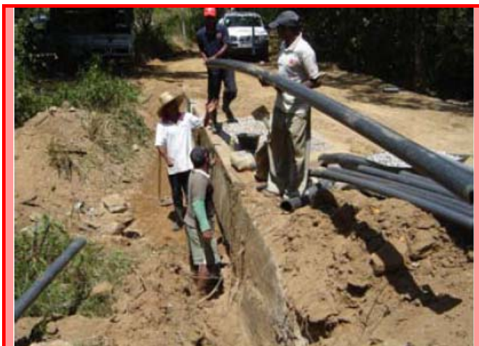
Labourers lay pipeline in the trench in Ampara district. Over 200 kilometres of new pipeline will bring piped water to 100,000 people living in Ampara district alone. German Red Cross.
