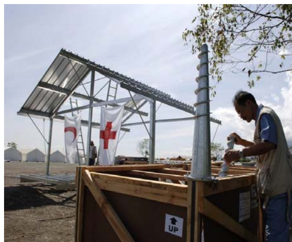
The construction of 20,000 steel-framed transitional shelters will provide improved living conditions for up to 80,000 of those worst-affected by the tsunami
