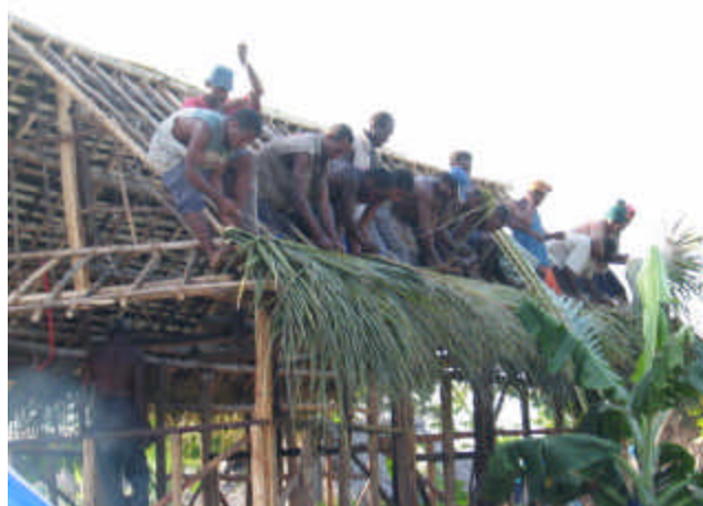
Communities in the care centres work together to construct shelters supported by the project.
