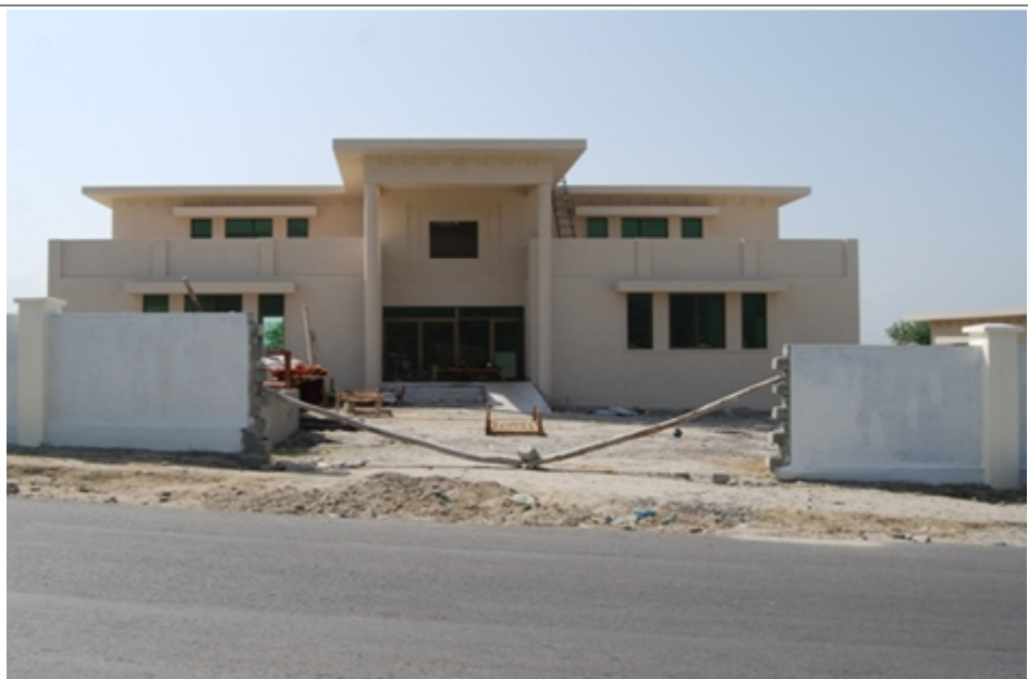
The branch office in Mansehra is largely completed, with only minor finishing works remaining. Photo: IFRC
