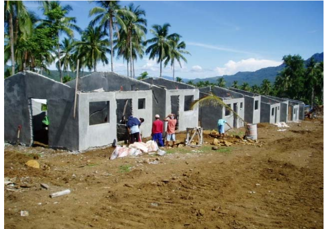
Some of the 60 duplex units in Catmon, St Bernard, in various stages of completion.
