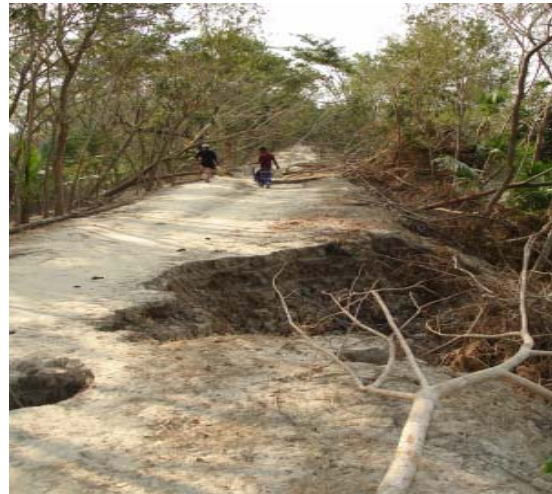
Badly damaged roads in Patuakhali district make travelling next to impossible
