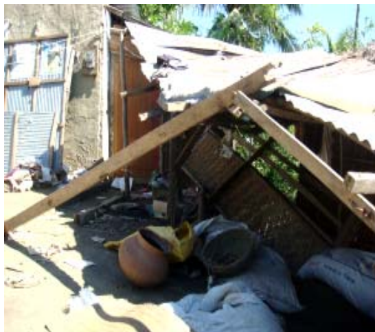
A house destroyed by Cyclone SIDR
