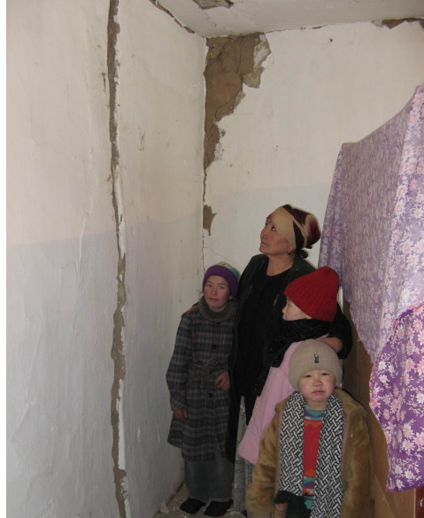
As time goes on, the damaged houses begin to collapse
