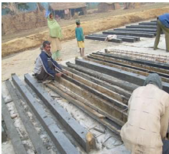
Houses being constructed in Hejarat village of Banke district, with NRCS support, for the relocation of 144 displaced families
