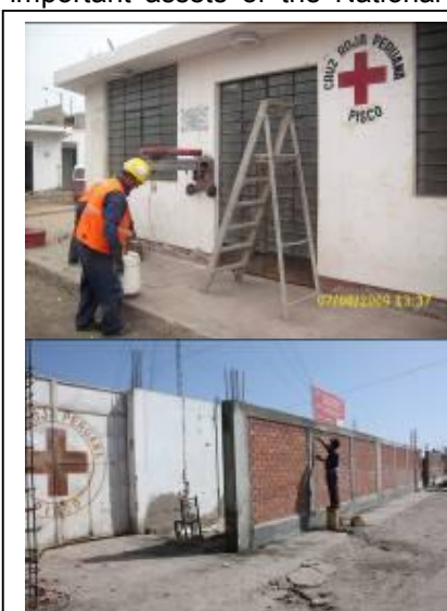
The operation has supported a dynamic assessment of the Pisco Branch existing infrastructure and the building of a new perimeter wall, which is currently ready. International Federation / P. Caveró & J. Ormeño
