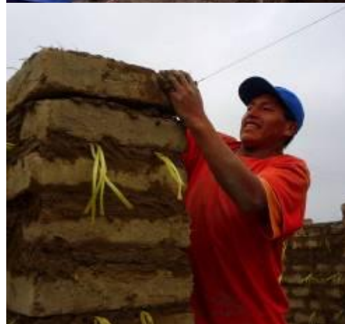
In Independencia (Pisco), members of the community take an active role in the building of their adobe houses. International Federation / J.Ormeño
